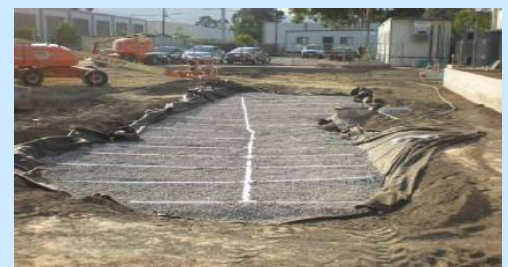
This underdrain pipe system will help to drain the bioretention area above it. Source: Brisbane City Hall, San Mateo County
