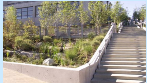
Stormwater from a rooftop drains into this terraced bioretention facility.
