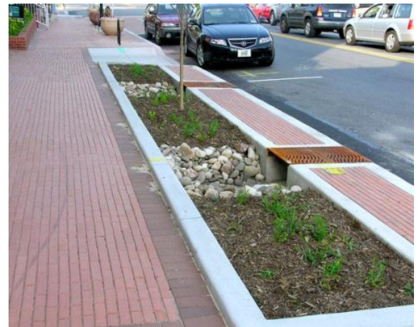
This roadside bioretention captures stormwater from the road. The paved shoulder and metal grates provide roadside parking access.
