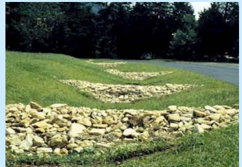
The rock check dams placed along this grassy swale help slow stormwater and prevent erosion in the swale (max. 6% slope).
